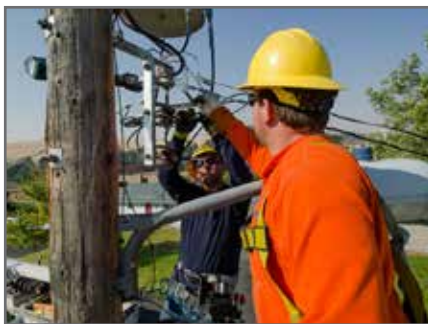
Avista installed smart transformers to help improve the efficiency of its distribution system in Pullman.
