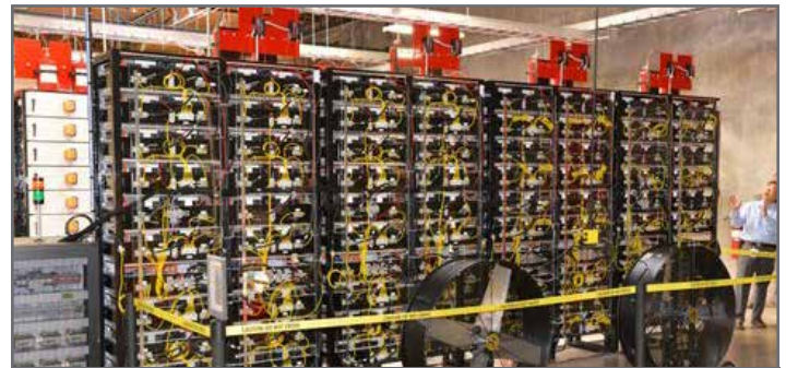
One of the PNW-SGDP highlights of the year was the May 2013 opening of the Salem Smart Power Center, which was partly funded through the PNW-SGDP. The photo shows a bank of batteries being tested at the center. Read more about this facility on page 9.
