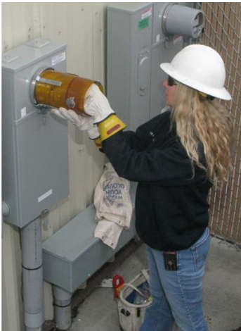
Automatic Meter installation at PNW-SGDP participant Flathead Electric
